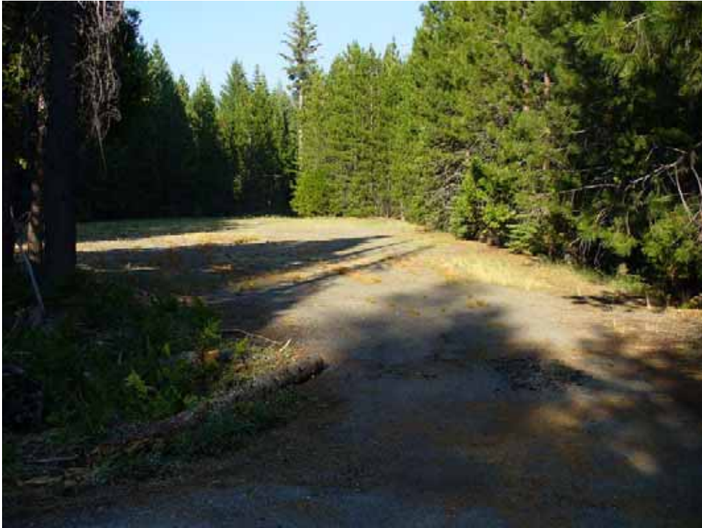
Photo P-2-9. South entrance to McGuire Boat Ramp Parking Area – northeast lot. Surface has deteriorated to base rock and is in poor condition. (7/23/08)
