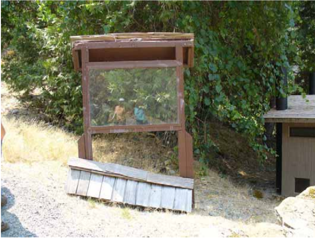
Photo T-2-9. Damaged information board adjacent to CXT upslope from parking area. (7/23/08)
