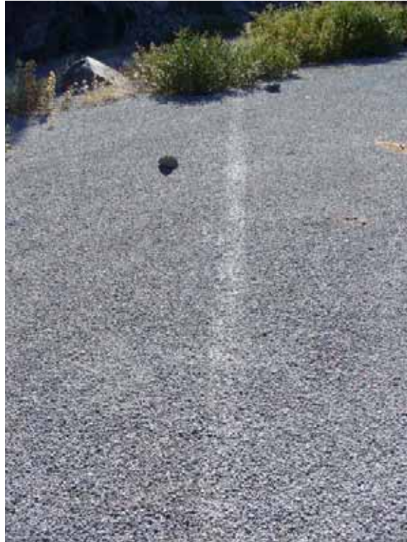
Photo H-2-26. Example of faded parking stall striping on asphalt with chip seal. (8/4/08)
