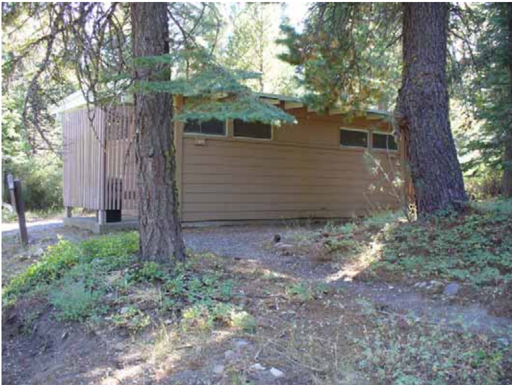
Photo K-2-12. Wood bathroom structure with flush toilets and sinks, not accessible. (9/04/08)
