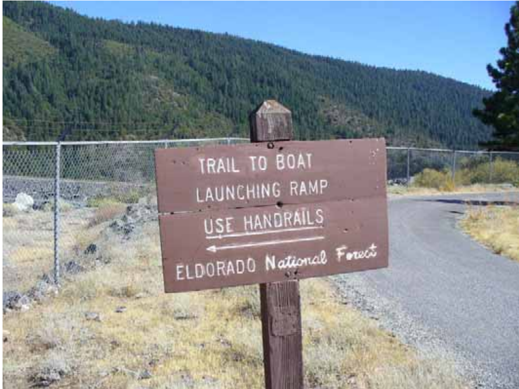
Photo H-2-30. Directional sign at entrance to trail/stairway to Hell Hole Boat Ramp. Sign is constructed of painted wood on wood post. Sign is in fair condition due to split boards and faded lettering. (8/4/08)
