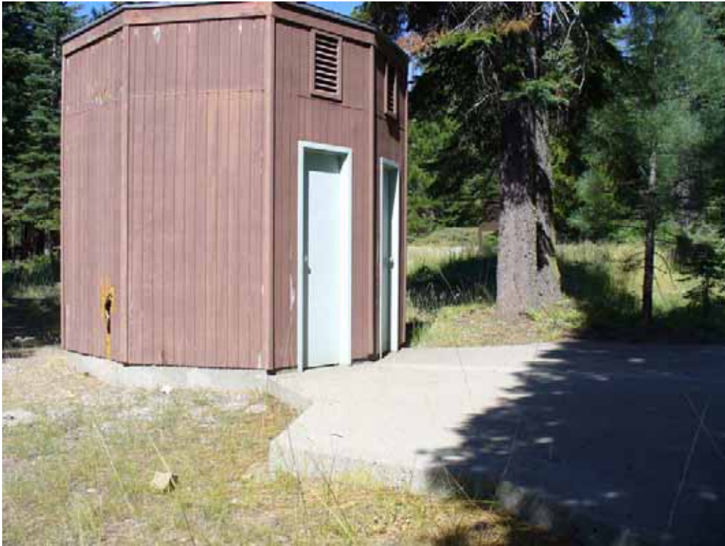
Photo Q-2-11. Backside of bathroom building. Space behind blue doors is now used for storage. Concrete pad was formerly a changing area. Note damage on building and large lip on concrete pad. (7/24/08)
