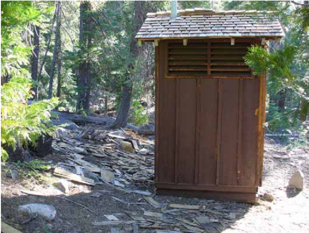
Photo L-2-15. Pit toilet side view. Note newly shingled roof and scrap shingles on ground. (7/24/08)
