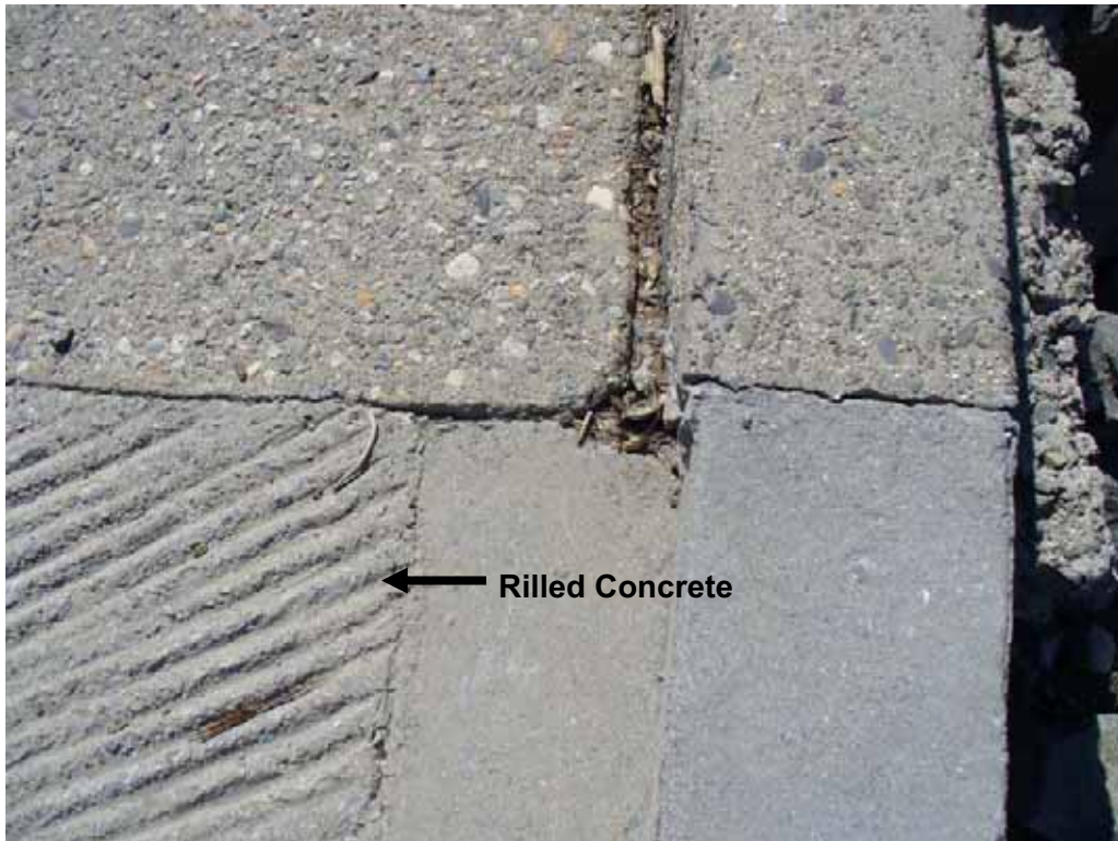
Photo H-2-5. Example of rilled concrete at lower end of ramp. (8/4/08)
