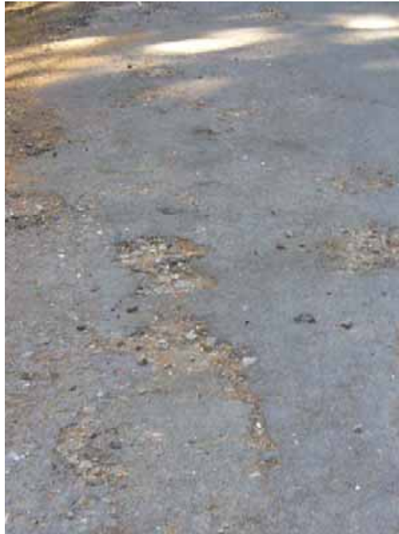
Photo E-2-7. Poor condition pavement at edge of Hell Hole Campground Parking Area. (8/21/08)
