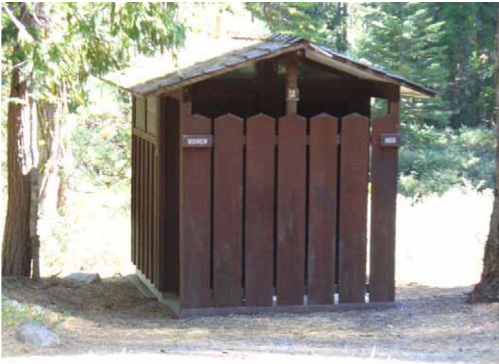
Photo K-2-10. Wood bathroom structure No. 2. This is a double unit vault toilet in fair condition. Not accessible. (9/04/08)
