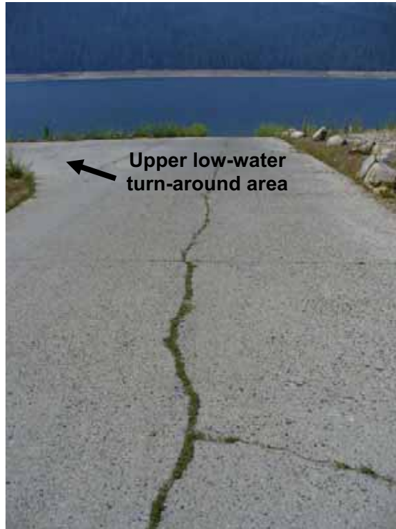
Photo O-2-2. Cracking in-filled with vegetation along French Meadows Boat Ramp, upper section. (7/23/08)
