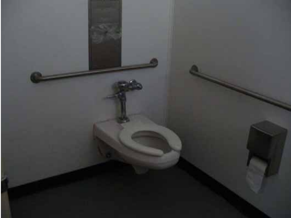
Photo K-2-18. Inside of wood bathroom structure converted to meet accessibility standards. (9/04/08)
