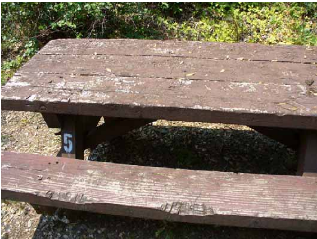
Photo S-2-6. Site 5 picnic table. Table is in poor condition and does not meet accessibility standards.
