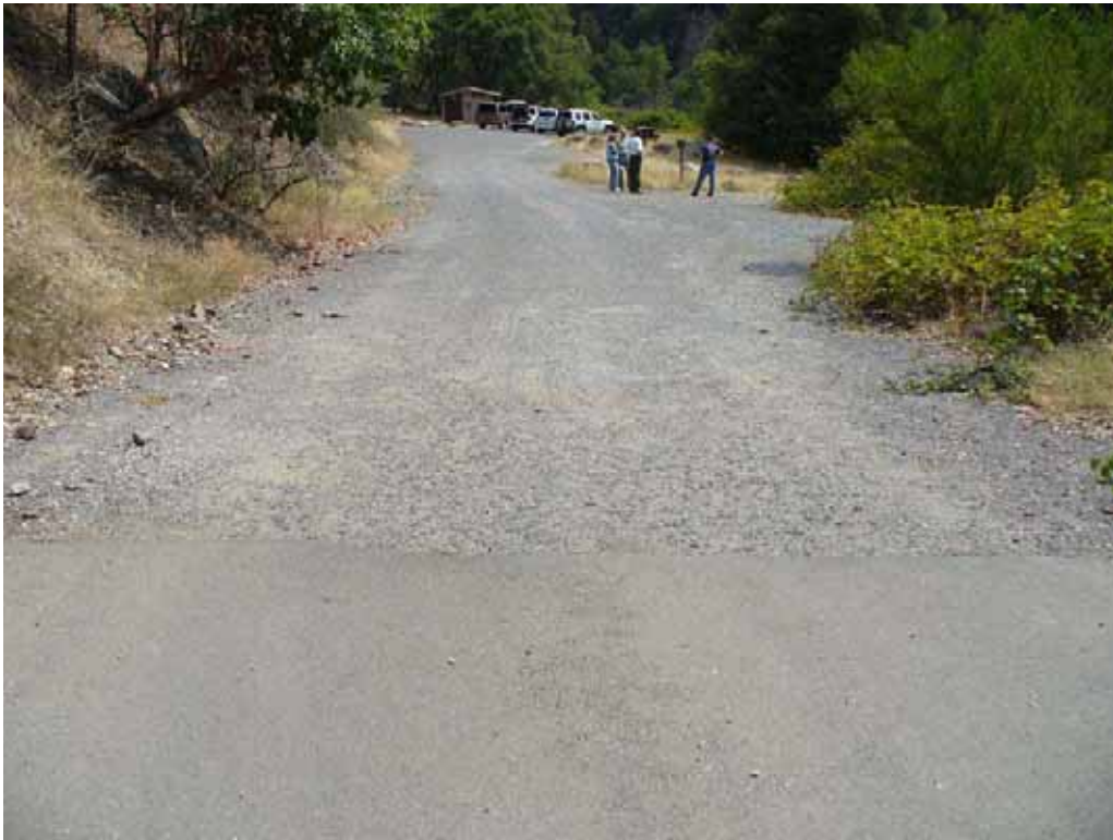
Photo S-2-2. Entrance to Ralston Picnic Area and Car Top Boat Ramp. (7/23/08)
