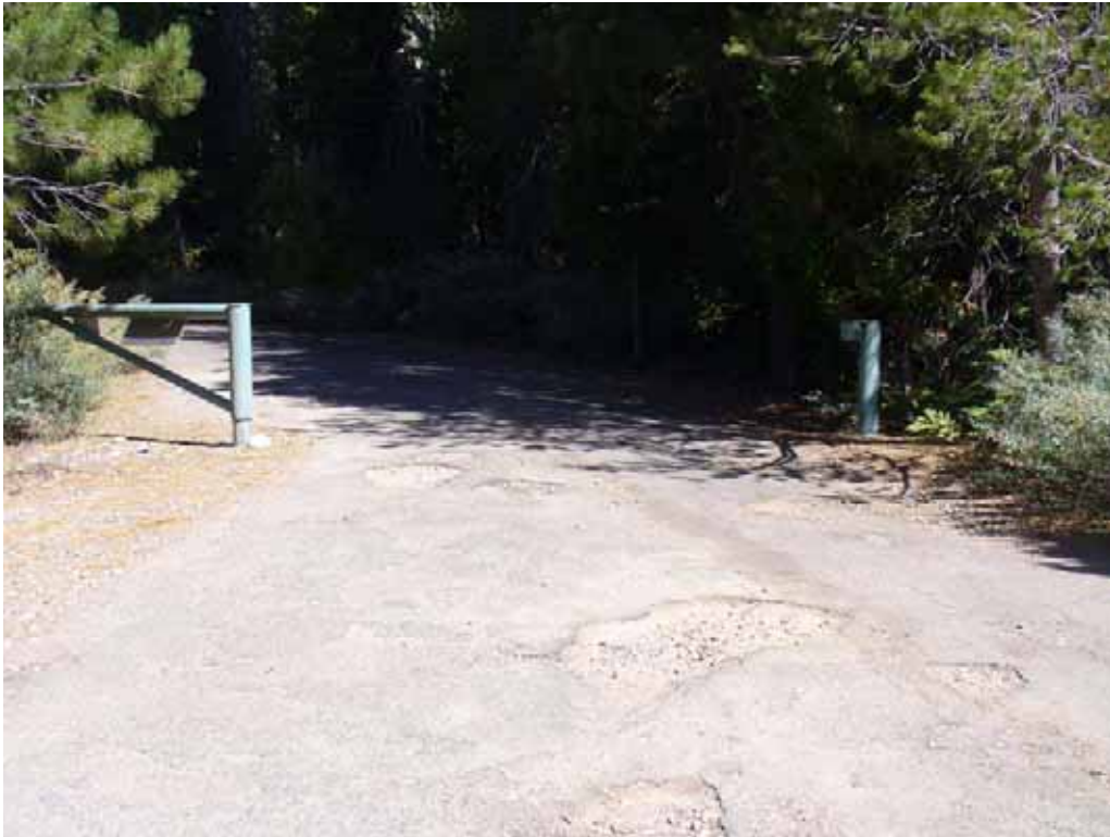
Photo D-2-3. Poor condition road surface at entrance to Big Meadows Campground. (8/21/08)
