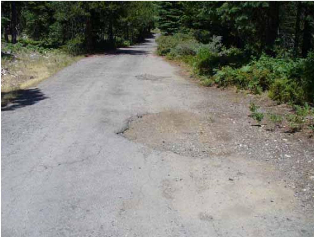
Photo Q-2-3. Potholes and damaged pavement along access road to McGuire Picnic Area, beach, and parking area. (7/24/08)
