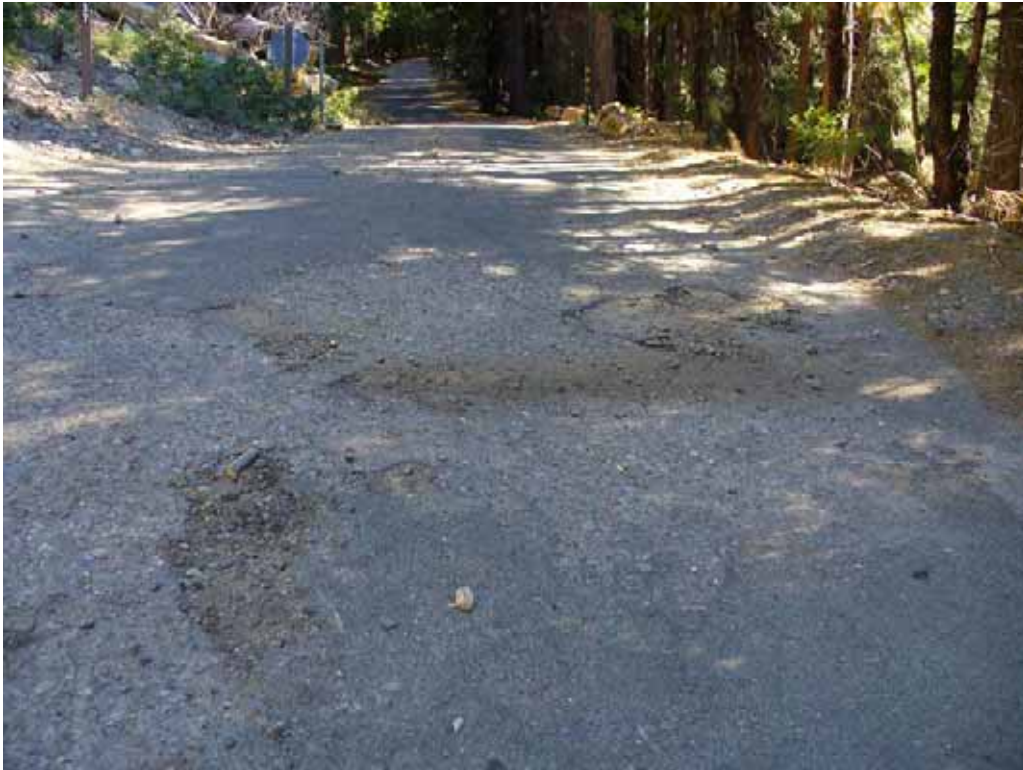
Photo E-2-3. Poor condition road surface at entrance to Hell Hole Campground. (8/21/08)
