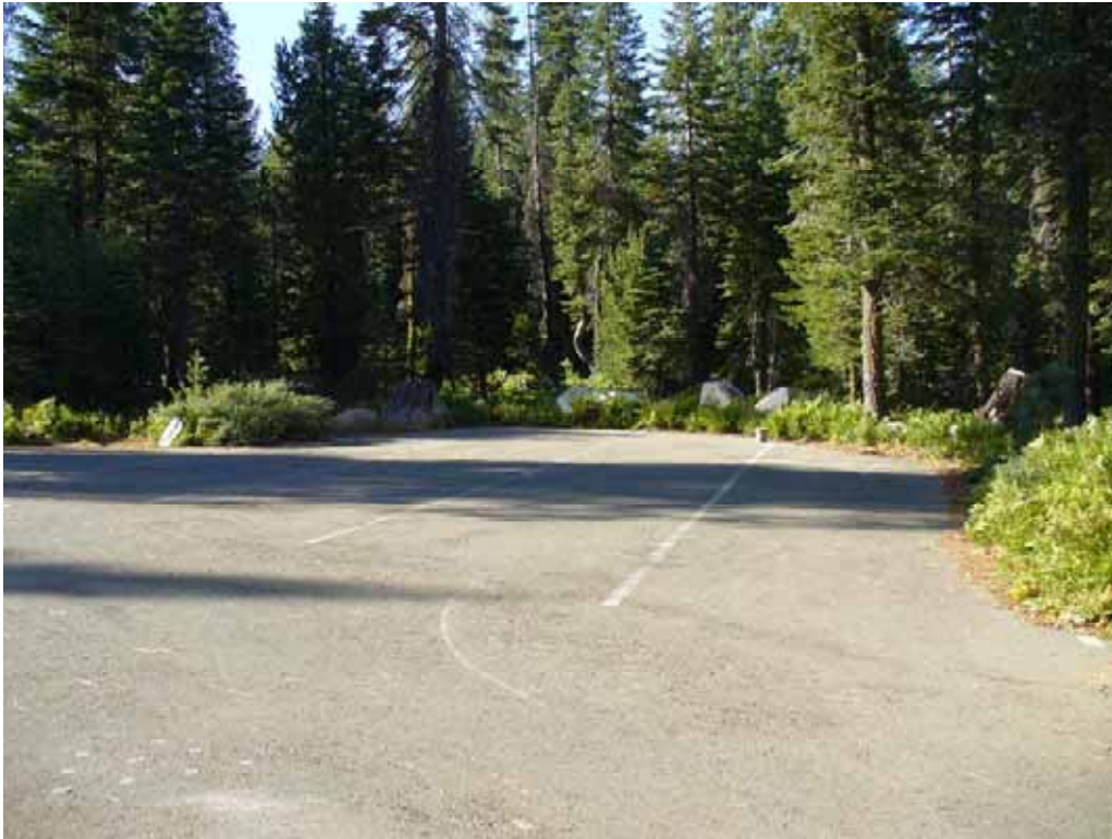
Photo N-2-7. Typical parking area at Gates Group Campground. This parking area is located at the entrance to Ponderosa. Note the striping and long stalls for trailers/RVs. Pavement is in good condition. (9/4/08)
