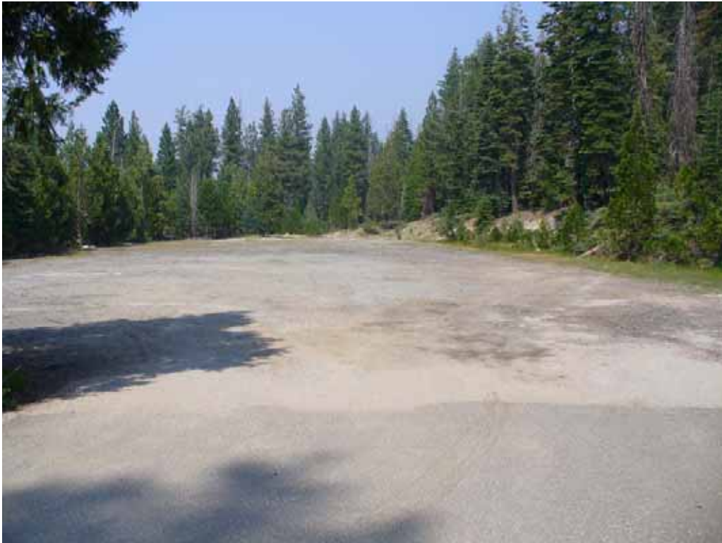
Photo O-2-5. French Meadows Boat Ramp Parking Area. Surface has deteriorated to aggregate base rock. (7/23/08)
