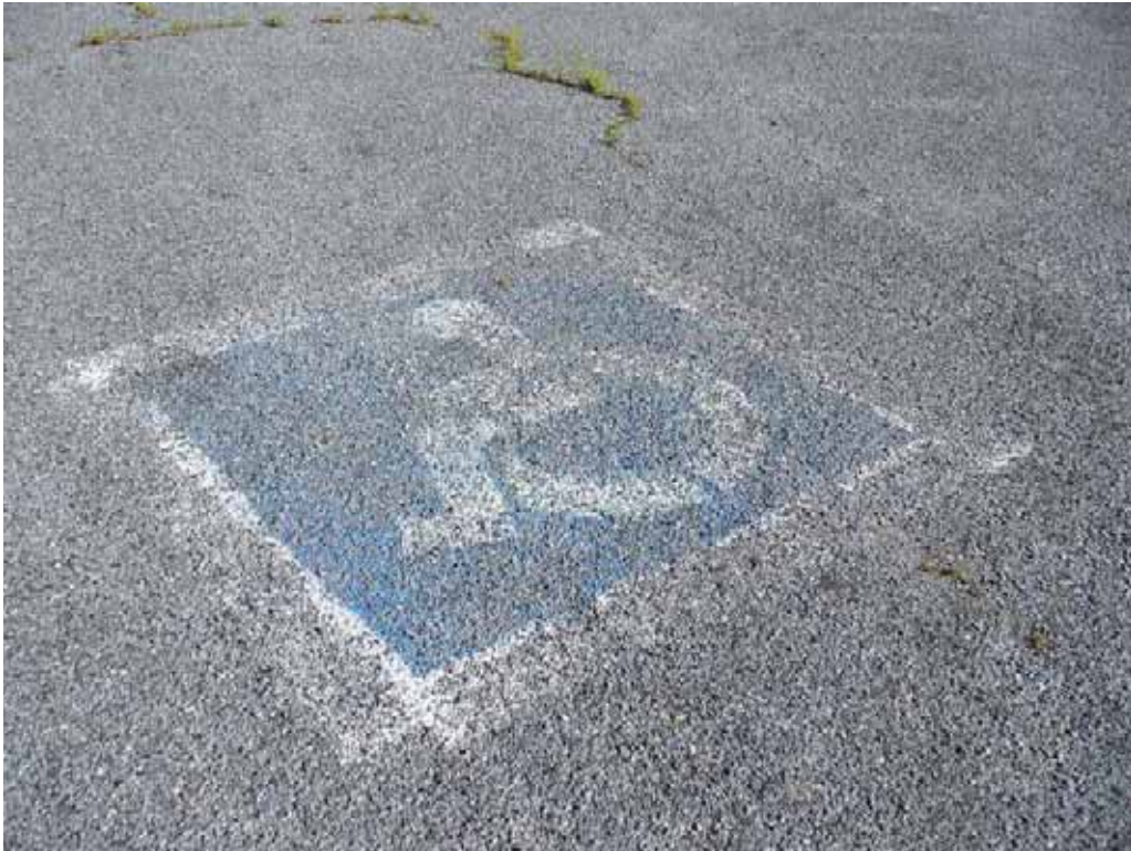
Photo H-2-25. Example of faded handicap parking area marking painted on asphalt with chip seal. (8/4/08)
