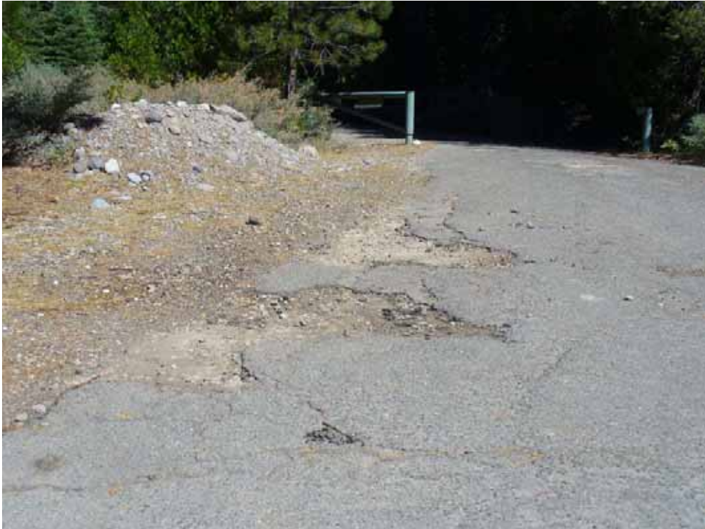
Photo D-2-4. Poor condition road surface at entrance to Big Meadows Campground. (8/21/08)
