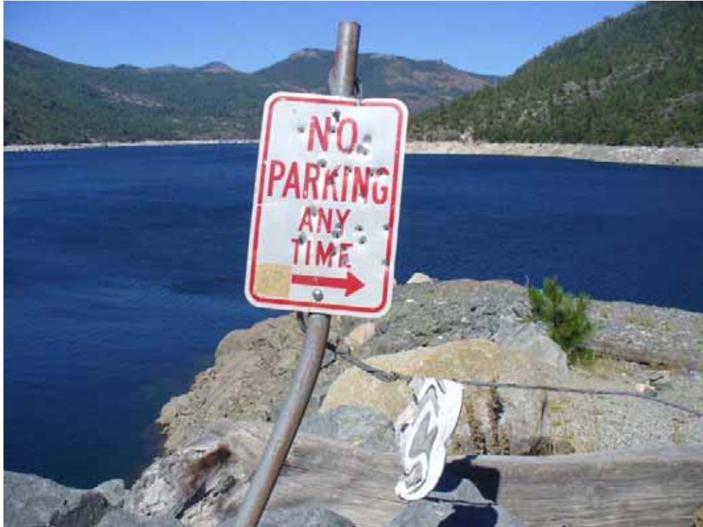
Photo H-2-16. Damaged "no parking" sign in lower lot. In poor condition due to bullet holes and bent steel post. (8/04/08)
