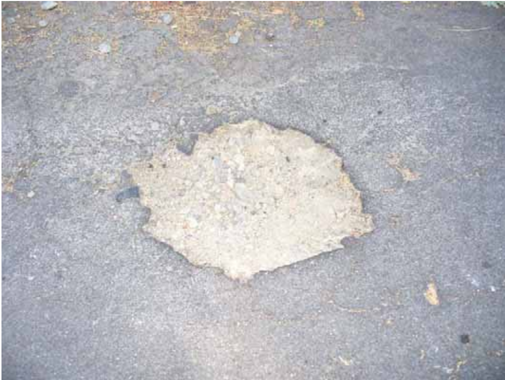
Photo E-2-5. Pothole in road near turn-out. (8/21/08)
