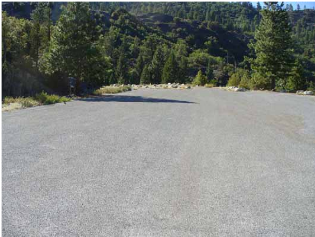
Photo H-2-22. Hell Hole Boat Ramp General Parking Area (northern portion). Surface is asphalt with chip seal in good condition. (8/4/08)
