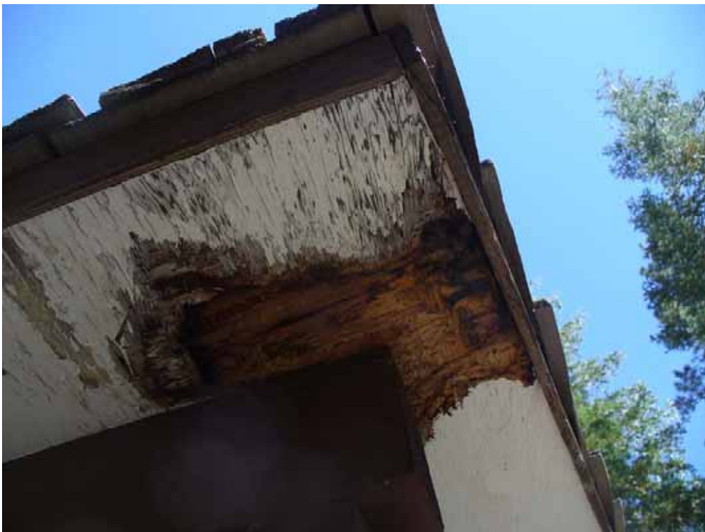
Photo I-2-14. Dry rot on roof and frame of toilet building No. 1. (9/04/08)
