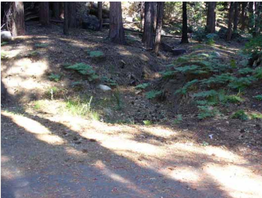
Photo E-2-10. Drainage into parking area. (8/21/08)
