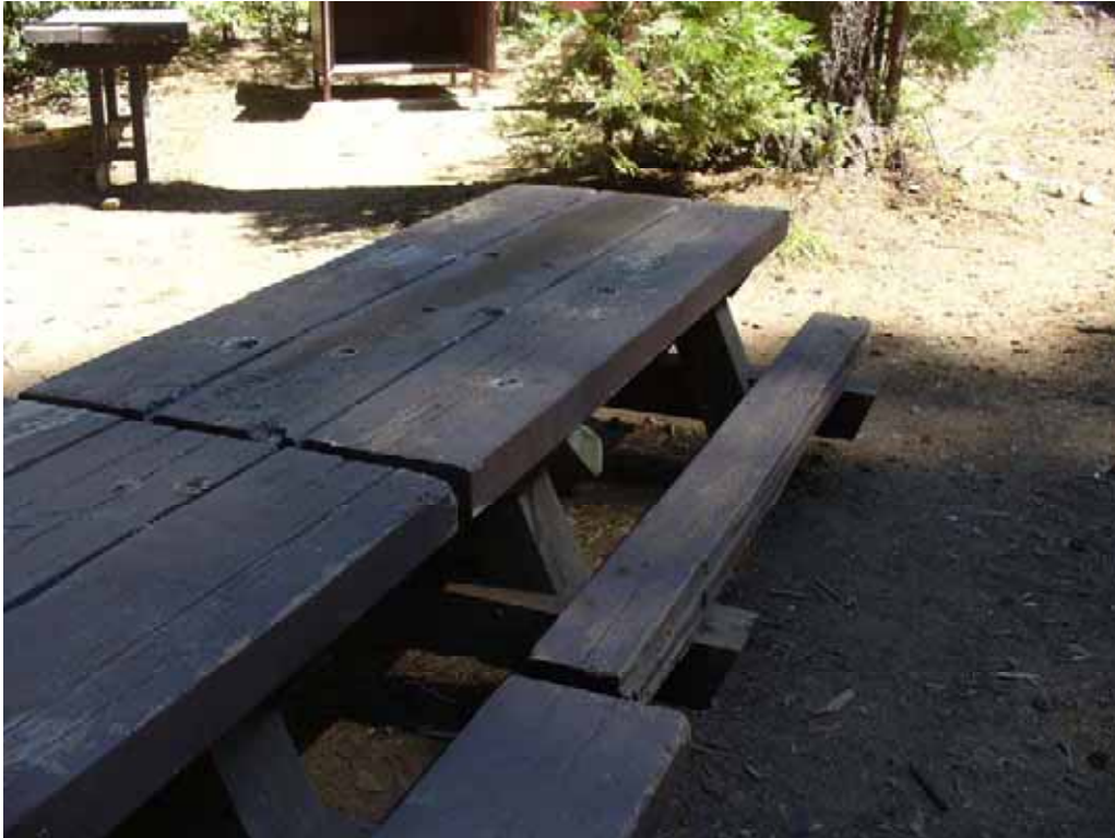
Photo R-2-12. Older picnic tables at Unit 1. All are in fair condition, with peeling paint and cracks. This one is in poor condition due to damage bench. (8/21/08)
