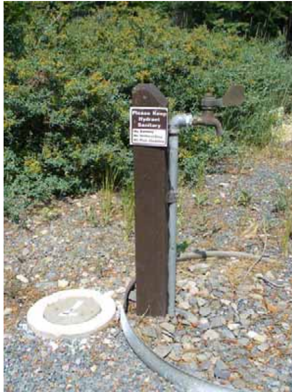
Photo O-2-11. Water faucet located adjacent to bathroom. Handle is considered disabled accessible. Approach is not disabled accessible due to insufficient clear space and changes in surface level. (7/23/08)
