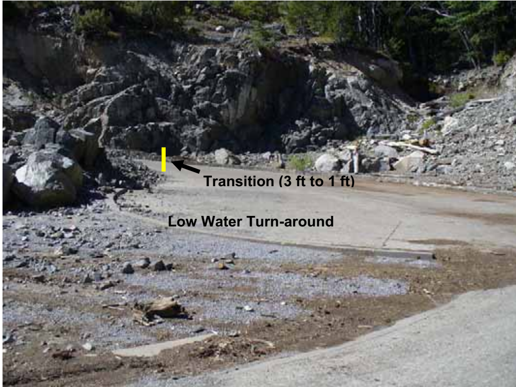
Photo H-2-4. Low water turn-around area in apex of ramp. Note that masonry retaining wall transitions from 3-foot high to 1-foot high. (8/4/08)
