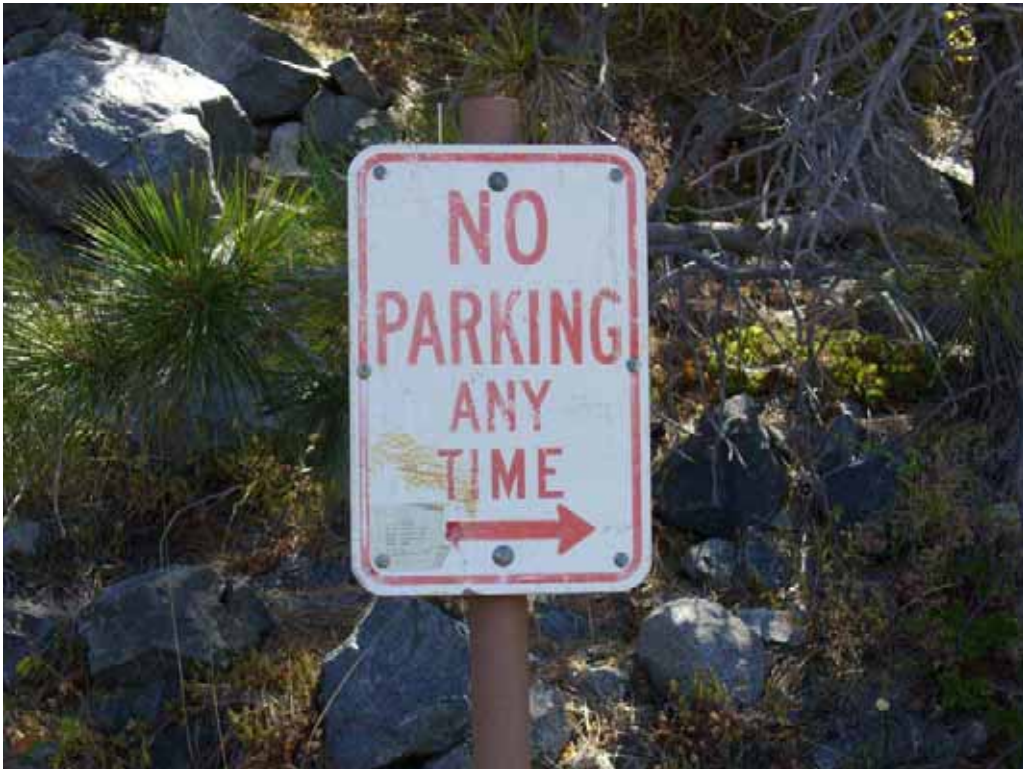
Photo H-2-2. Example of “no parking” sign located along Hell Hole Boat Ramp. Condition is “fair” due to faded lettering. (8/4/08)
