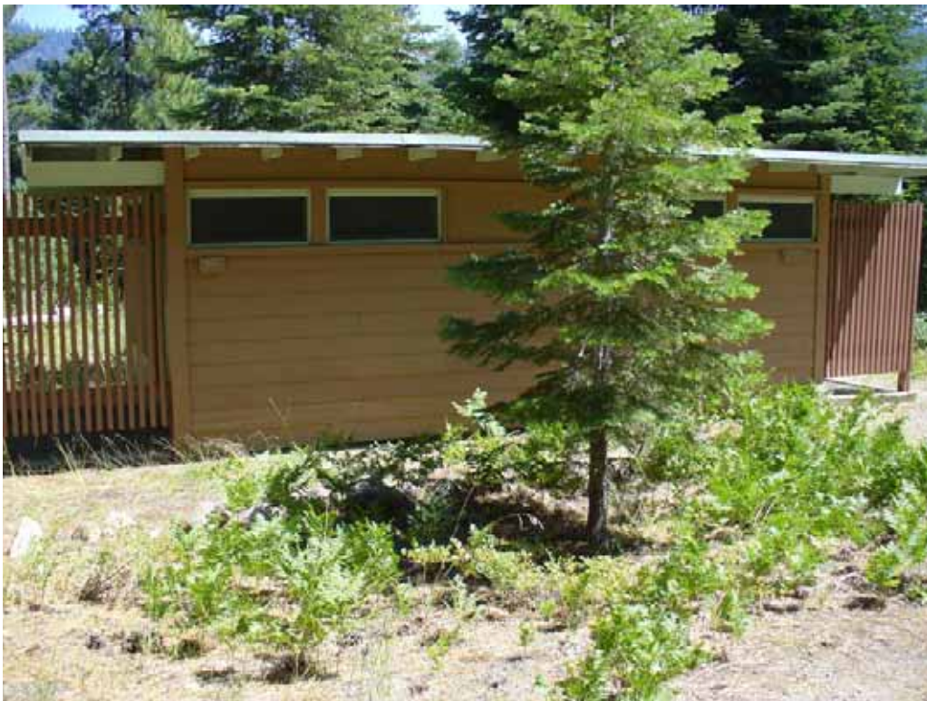
Photo Q-2-6. Bathroom located adjacent to parking area. Not disabled accessible. (7/24/08)
