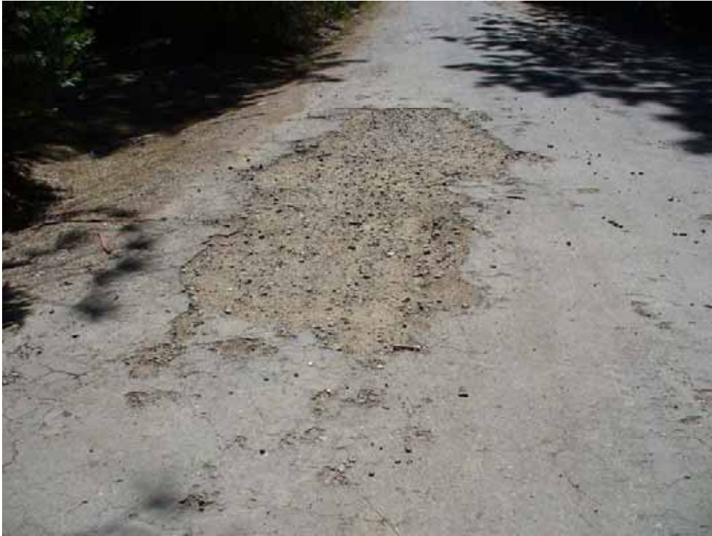
Photo R-2-3. Example of poor condition pavement along Middle Meadows Campground Access Road (14N28). (8/21/08)
