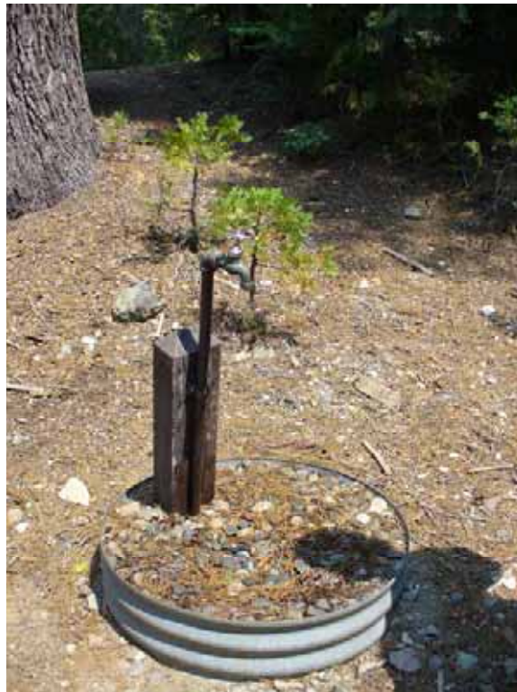
Photo O-2-18. Water faucet near vault toilet. Does not meet accessibility standards due to handle design, obstacles, and level changes. (7/23/08)
