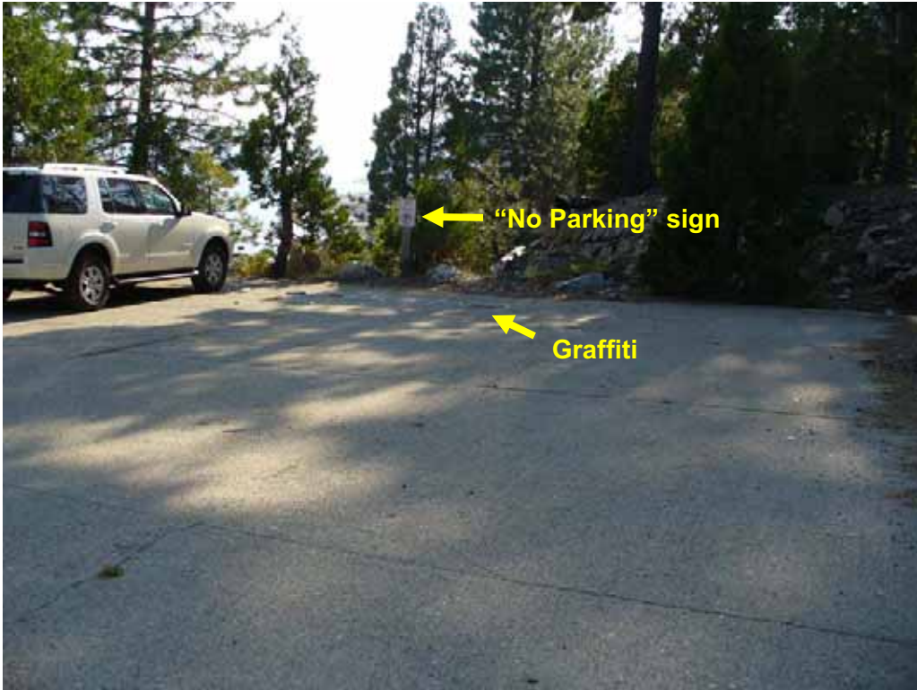
Photo P-2-3. High water turn-around and loading/unloading area. Note “no parking” sign and graffiti on surface. (7/23/08)
