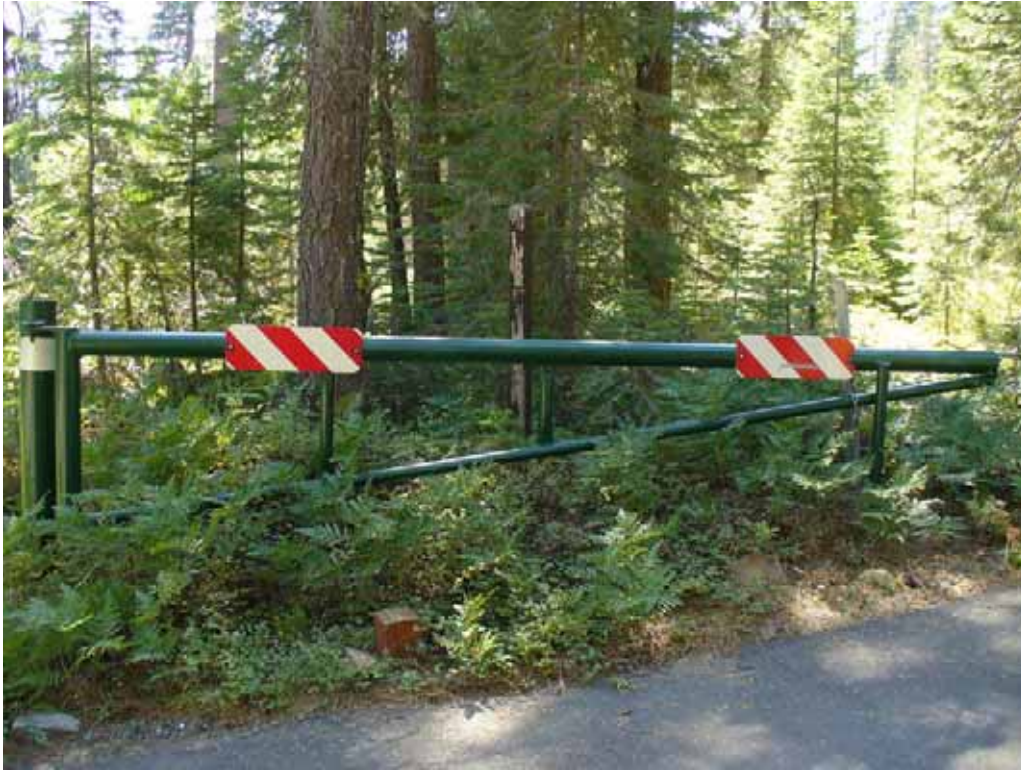
Photo K-2-3. Swing gate with reflective hazard signs located at entrance to Lewis Campground, good condition. (9/04/08)
