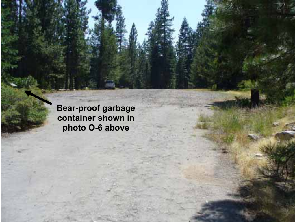
Photo Q-2-4. McGuire Picnic Area and Beach parking area. Note deteriorated asphalt surface. (7/24/08)
