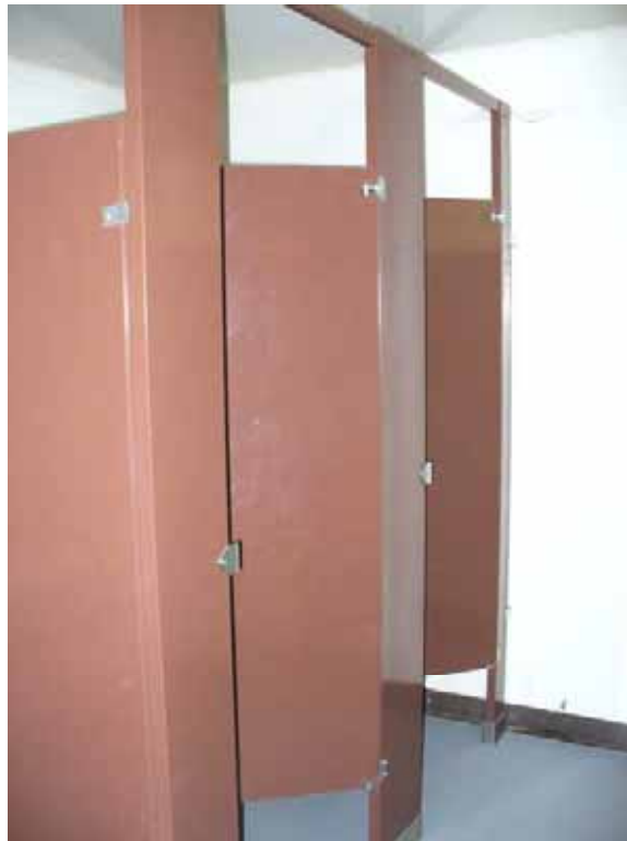
Photo K-2-14. Stalls inside of wood bathroom. These stalls are not accessible but this type of bathroom can be converted to meet accessibility standards. (9/04/08)
