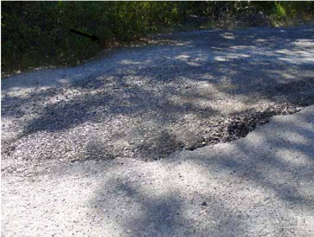
Photo G-2-3. Example of damaged pavement surface in Hell Hole Vista Parking area. (8/20/08)
