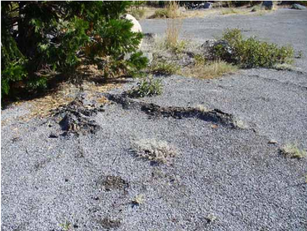
Photo H-2-27. Example of damaged surface in southeastern portion of parking area. (8/4/08)
