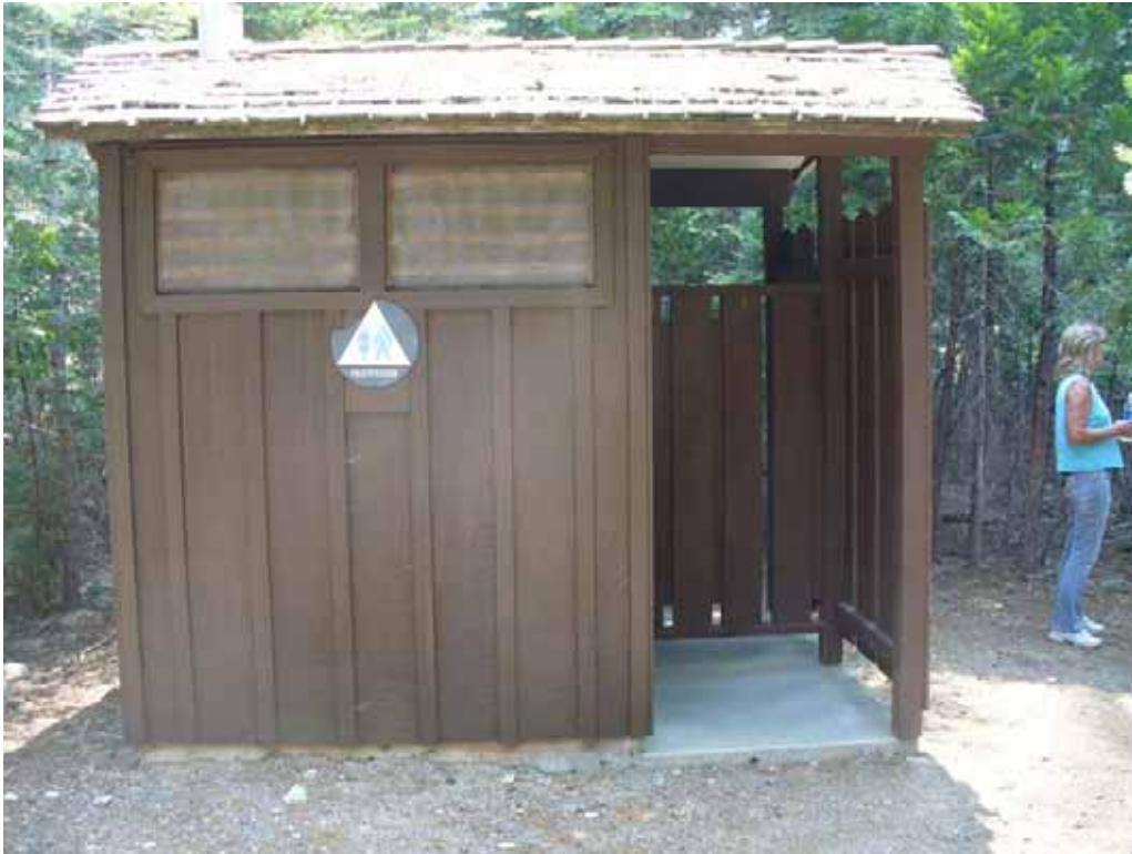
Photo O-2-17. Two-unit vault toilet located in French Meadows Picnic Area. This toilet does not meet accessibility standards due to narrow entrance width, level changes (e.g., concrete lip) and absence of hand rails. (7/23/08)
