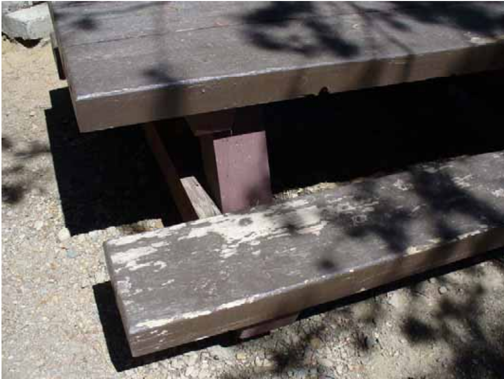
Photo I-2-11. Typical heavy wood table showing flaking paint. (9/04/08)
