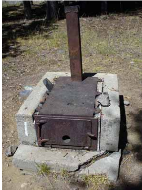
Photo I-2-7. Concrete and steel stove at site 1, poor condition. (9/04/08)
