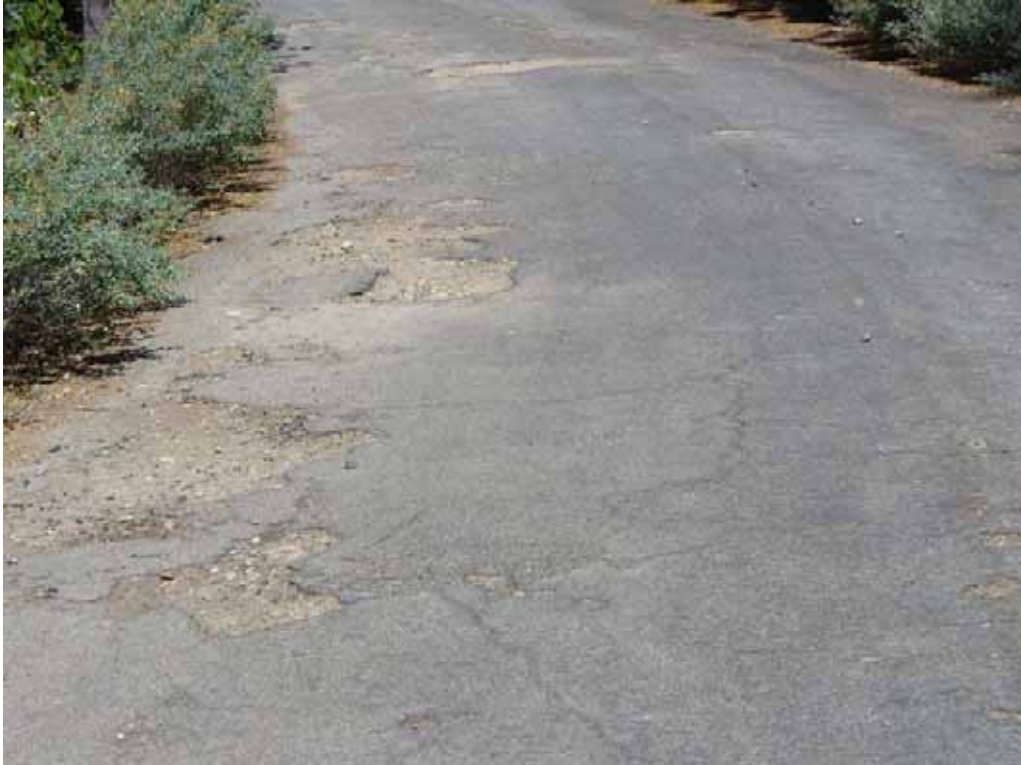
Photo D-2-6. Poor condition pavement along 14N43, the access road to Big Meadows Campground (8/21/08).
